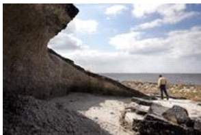
Lake Okeechobee just south of Pahokee where the dike was damaged by erosion after Hurricane Wilma.
